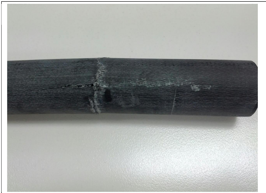
E-glass. Rough tears can be seen where the break has occurred. This is evident on the full circumference of the stanchion.
