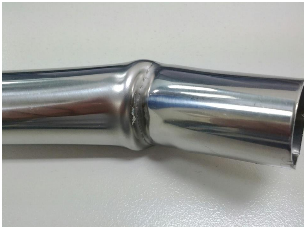
Stainless Steel. The tear can be seen in the middle of the fold. Straightening the stanchion risks breaking the stanchion in half.
